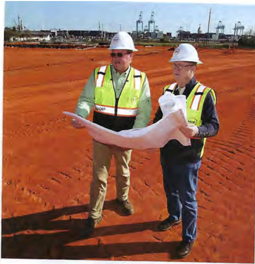
Giles and Royster review plans for the structure slated to open late this year.
